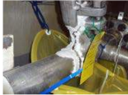
Boric acid leak in a nuclear plant.
